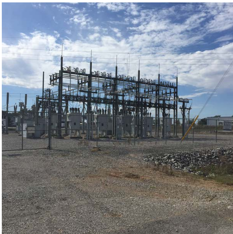
Figure 7 Industrial Park Electric Substation
