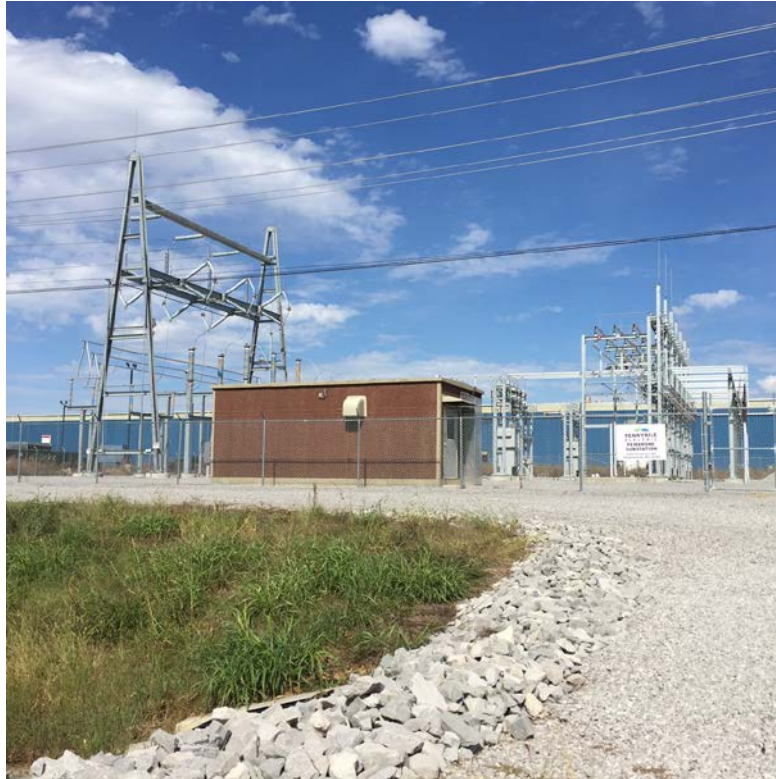
Figure 6 Pembroke Road Electric Substation
