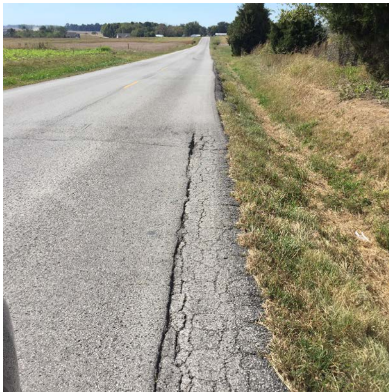
Figure 5 Pavement/ subgrade failure, common on KY 115
